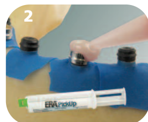
2. Add ERA PickUp® Material over the top and sides of the metal jackets.
